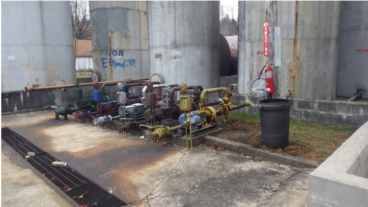
ASTs refill area with release catch basin.
