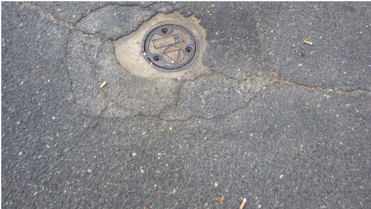
Monitoring well (not secured)
