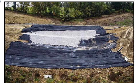
Installation of geotextile fabric for soil separation and stabilization – image from Foundation Geotextiles website
