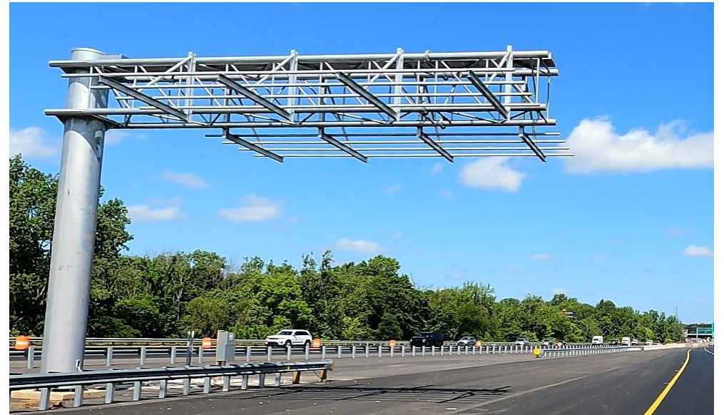
Express lane gantry at Site 1
