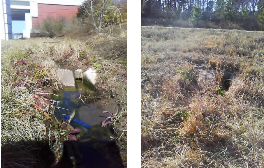
Figure 3: Miscellaneous Drainage Inspection Results Sample
