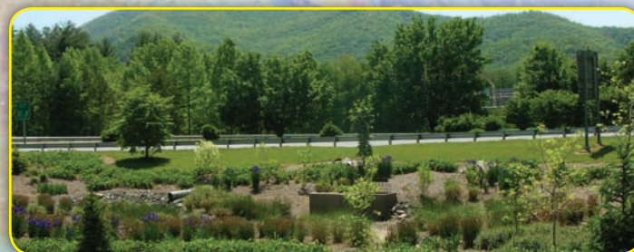
Left: NCDOT dry detention basin installed near Dillsboro captures stormwater runoff and allows time for the ground to adsorb it.
