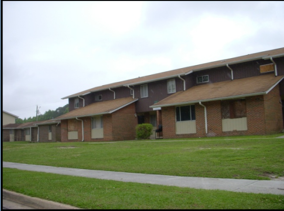
A HUD Housing Development along 30 th Street where some of the units have been abandoned.
