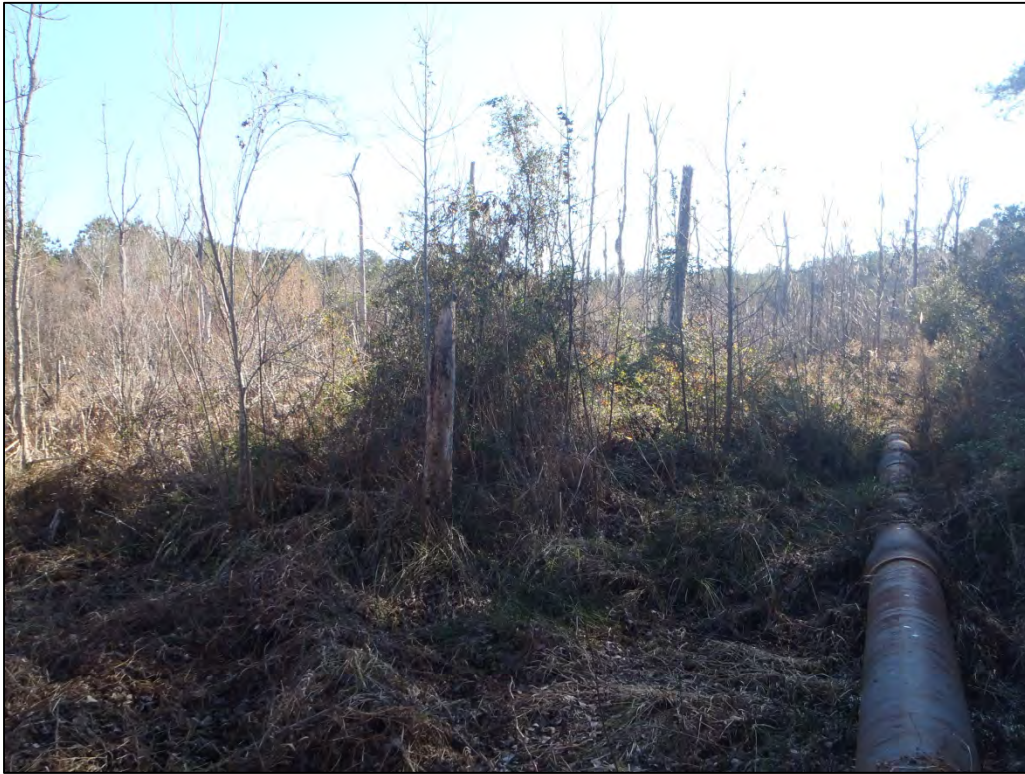
CROSSING 1, EXPOSED SANITARY SEWER LOOKING EAST
