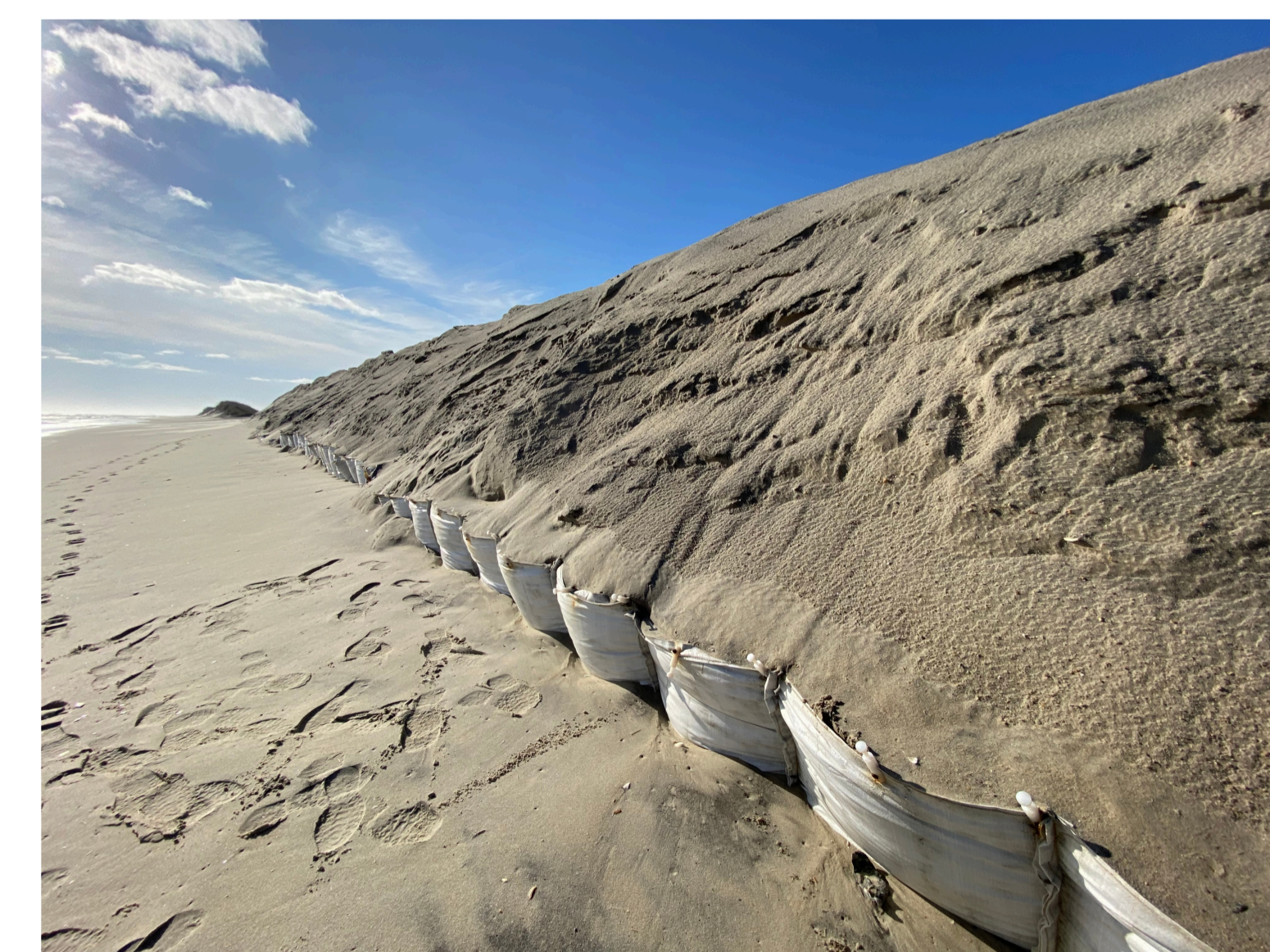
An engineered shoreline stabilization effort implemented to protect dunes and infrastructure. The sand-filled barriers are used as a temporary measure to slow coastal erosion caused by waves, storms, and rising water levels.
