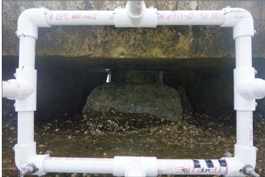
Photo 16. Representative photo of concrete substrate for a middle elevation monitoring station (Station 7) showing wet concrete, algae, and barnacle growth on the structure at the Bonner Bridge Seagrass Mitigation Site during the May 2019 survey.
