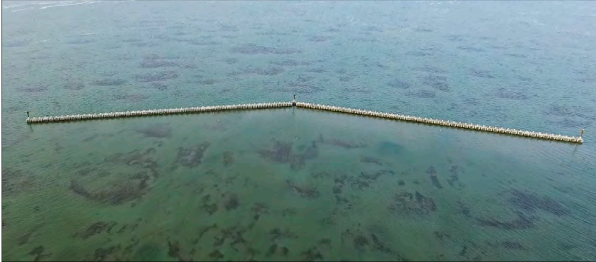
Photo 18. North-oriented view of the wavebreak installed in January 2017 at the Bonner Bridge Seagrass Mitigation Site. The total structure length is 500 ft (152 m).
