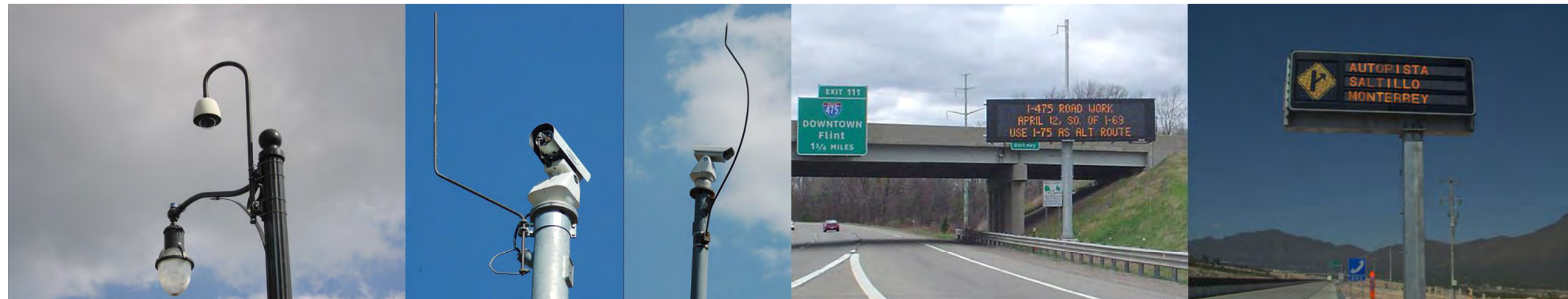
Examples of pole-mounted closed circuit television cameras and dynamic message signs
